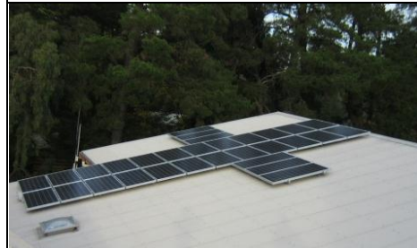
PV Panels on Roof
