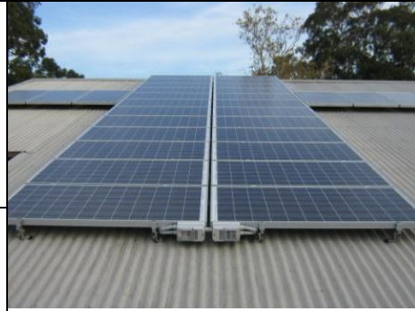
PV Panels on Roof
