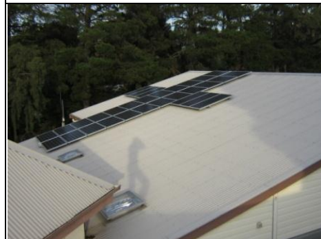
PV Panels on Roof
